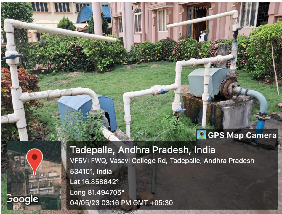
Fig. Borewell water saved in tank and supplied to RO unit for purification
