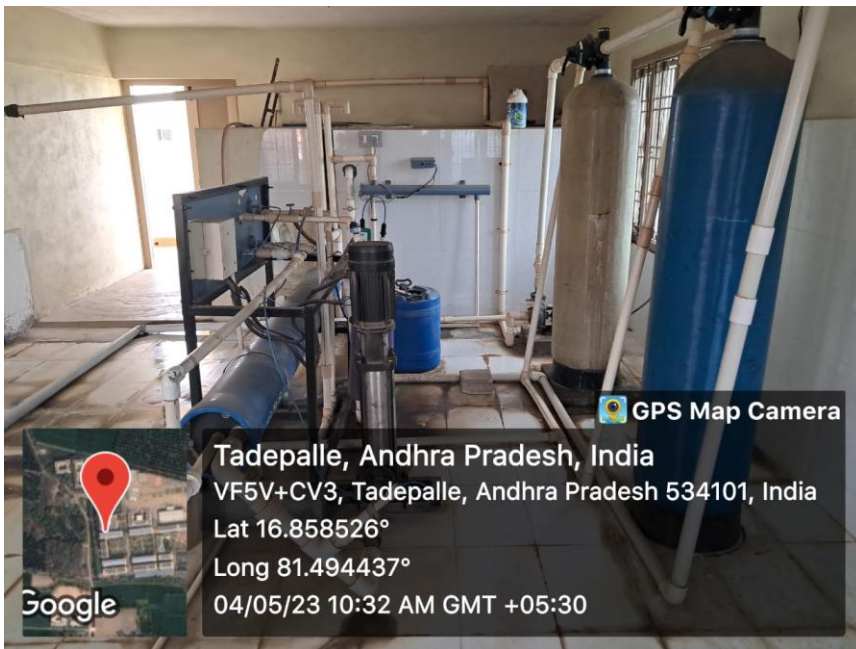
Fig. RO PLANT at ECE D block third floor.
