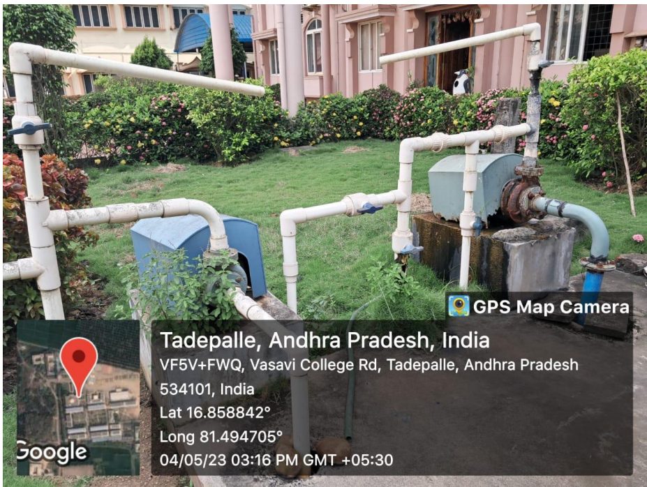
Figure Borewell water tank with sump
