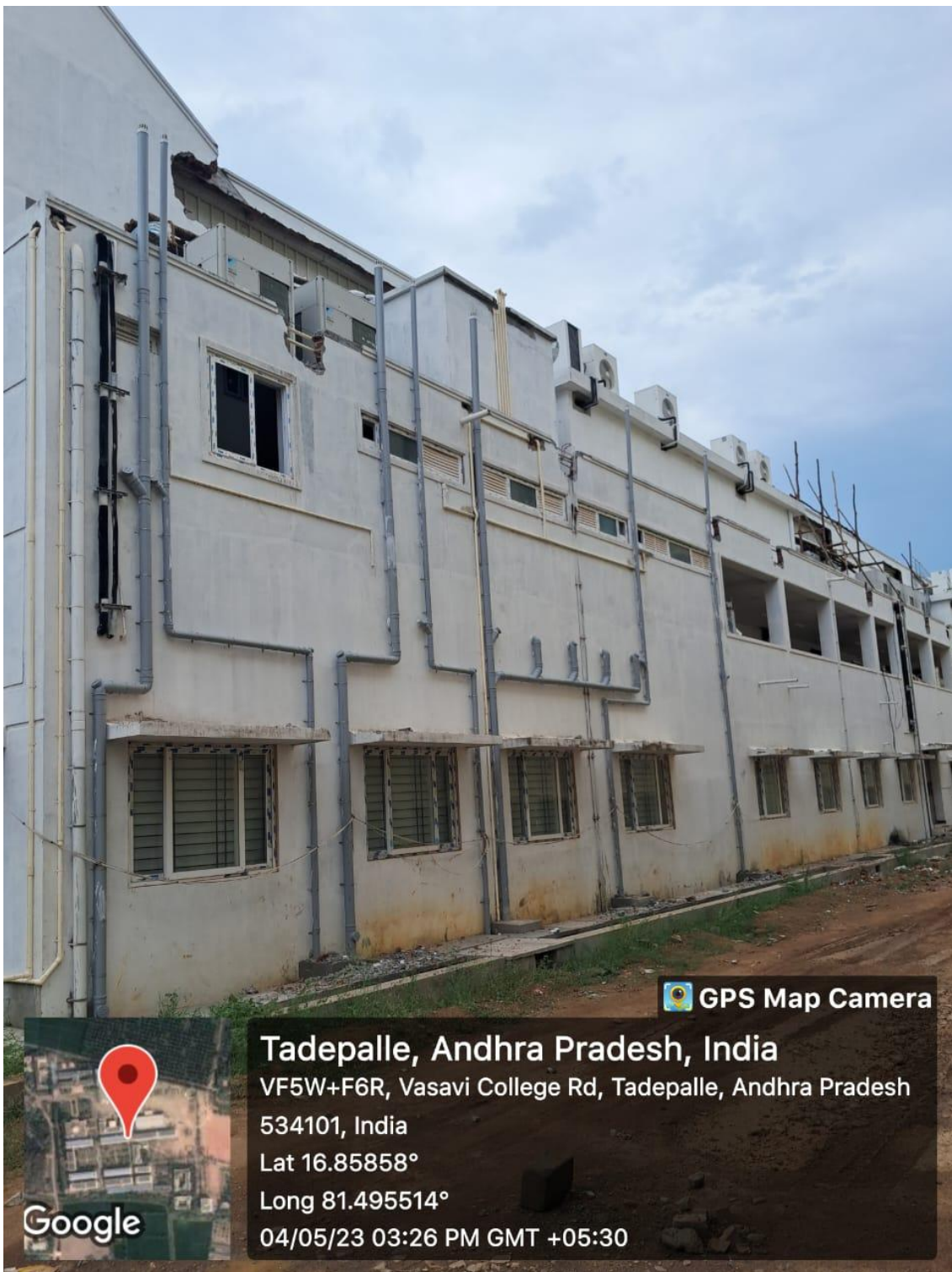
Fig. Water distribution pipes in Auditorium block
